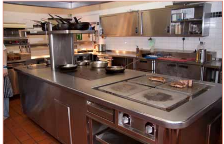
This French made Athanor range is designed specifically for cooking and holding top quality steaks. Both Ramside Hall and Hardwick Hall have these ranges in their Rib Room kitchens.
